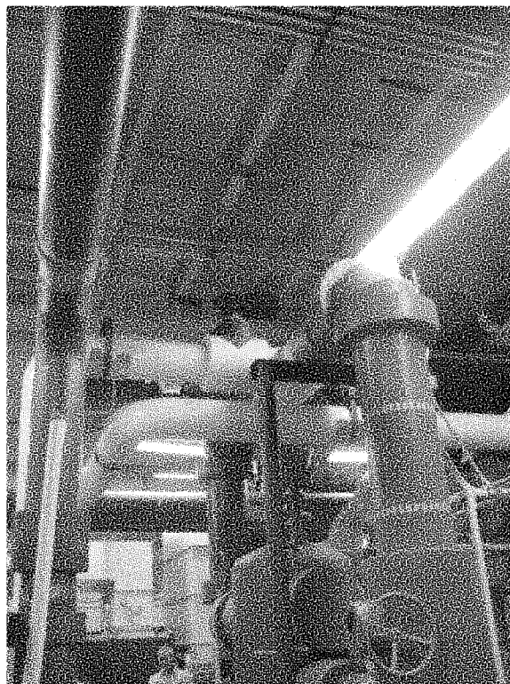
Branch Connection Missing
