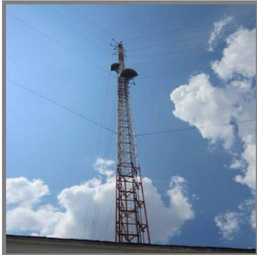
Celina Guyed Radio Tower
