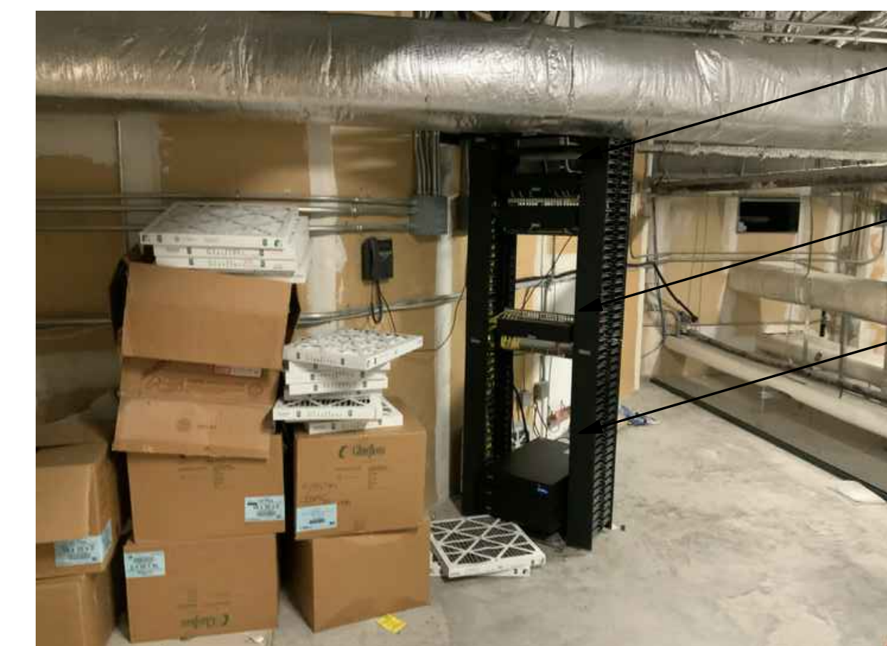
1A EQUIPMENT PHOTO
