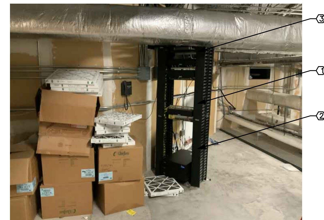
1A EQUIPMENT PHOTO
