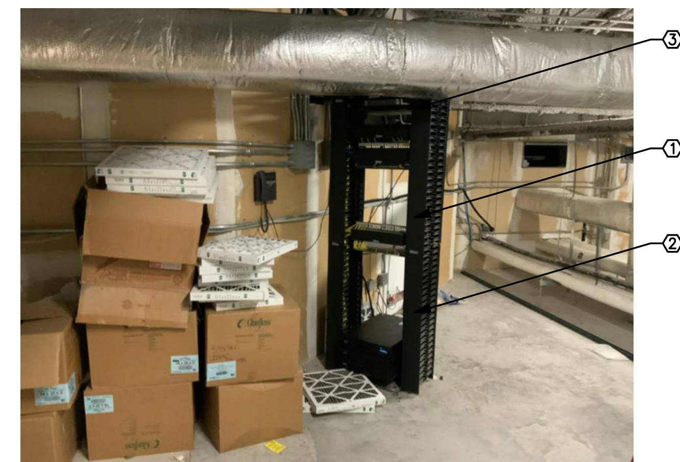
1A EQUIPMENT PHOTO
