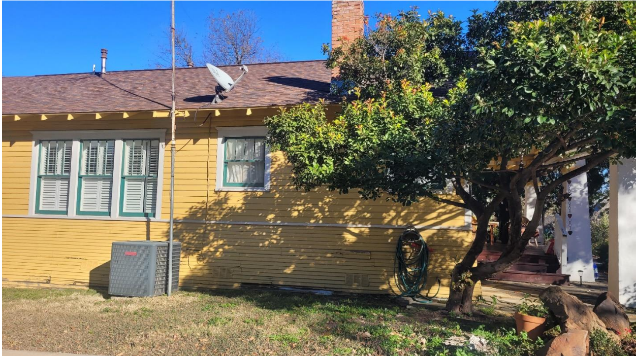
Twin Bungalow 408 West Heard Street McKinney Lots of rotten wood
