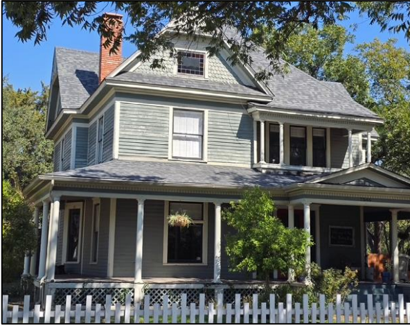
Dow Baccus House: Residential 7546 Oak Street, Frisco, Texas Peeling paint on exterior, rotting wood
