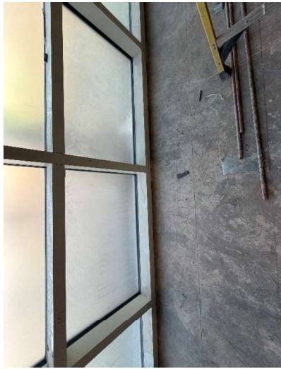
Photo 4: Water testing sill
